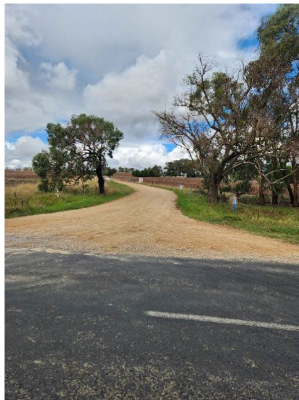
Photograph 6: Wear on Edge of Pavement at Junction of Property Access and Old Forbes Road
